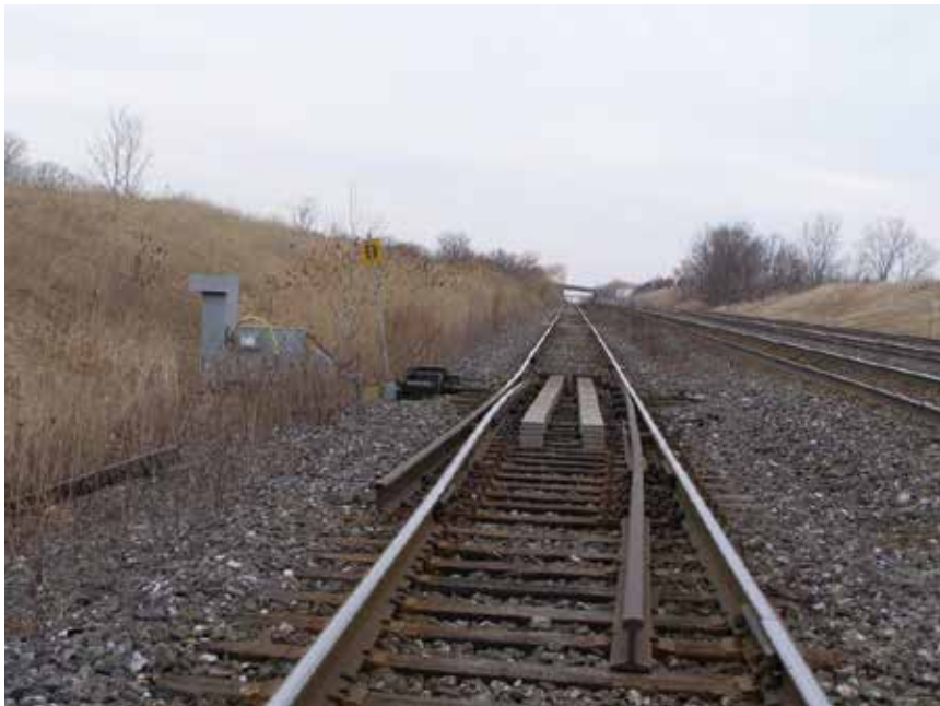
Photo 2. A switch point derail operated by a power switch
