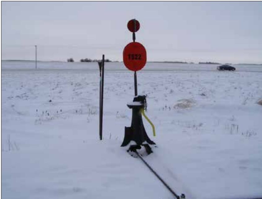
Photo 1. Mainline track switch TS 22 in the normal position
