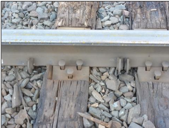
Photo 6. Anchors situated away from the tie
