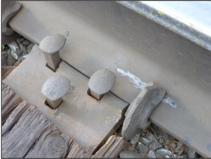
Photo 7. Anchor abrasion markings on the rail base
