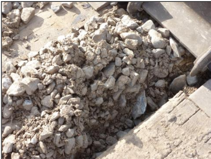
Photo 13. Fouled ballast being plowed by the tie
